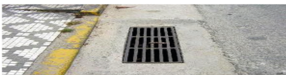
Figure 4: Manhole with grill
