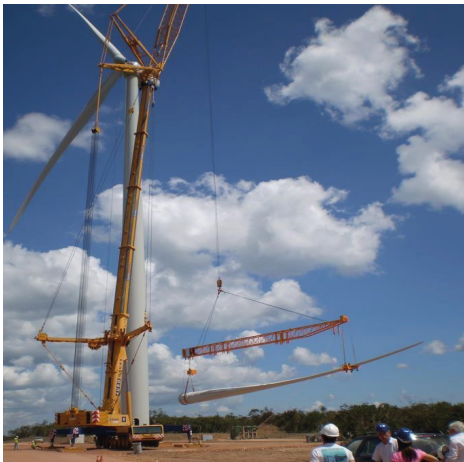
Figure 04: Assembly of the 1st Wind Farm in Bahia in Brotas de Macaúbas, March 31, 2011.
