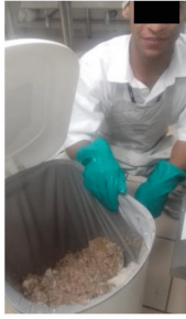
Figure 1 – Food crusher installed in the restaurant pantry
