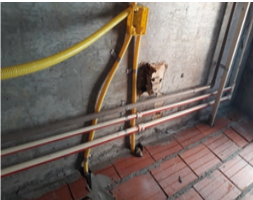
Figure 6 – Pipes installed and fixed without bends - Tower B.
