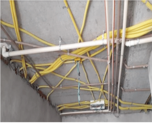
Figure 5 – Pipes installed and fixed under stress, in Tower A.
