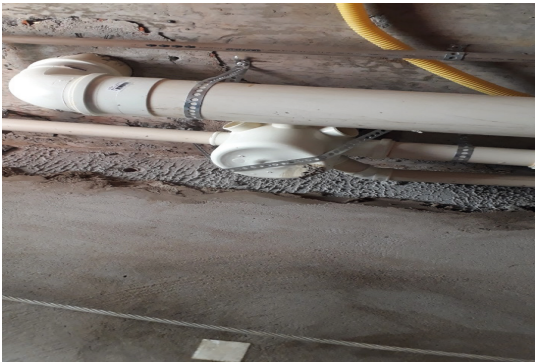
Figure 3 – Siphon box fixed with metal tape.
