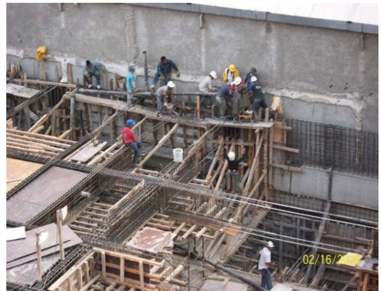
Figure 2: Unsafe scaffolding conditions.
