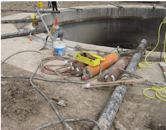
Figure 1: Excavation without guardrail and general disorder. Own source.
