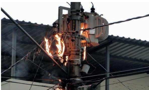
Figure 1 – Power transformer in electrical grid distribution
