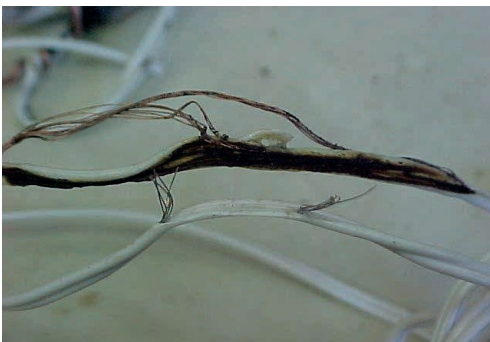
Figure13 – Conductors after being subjected to overvoltage.
