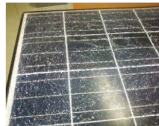
Figure 4. Photovoltaic module presenting glass breaks (Ndiaye, 2016)
