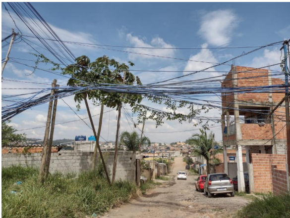
Figure 3: Clandestine connections hoses. Source: Sabesp (2022)
