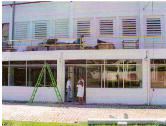
Figure 2: View of the lower and upper floors of the Ground floor slab panel to be analyzed
