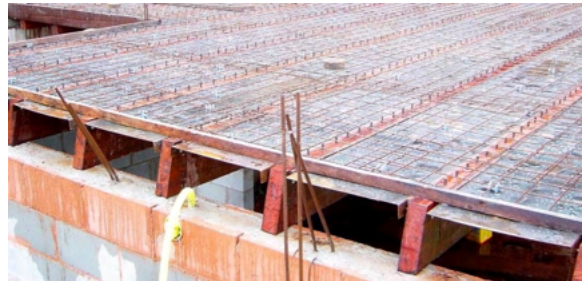
Figure 7 - Mixed structure of concrete slab cast in loco on the wooden beams, supported at the wall of masonry-Source:personal archives
