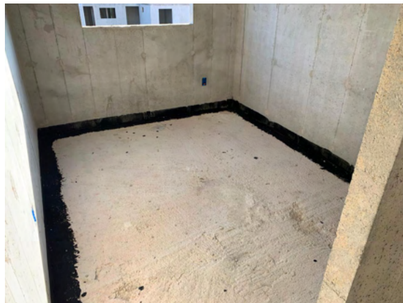
Figure 3 - Application of acoustic blanket adhered to the entire perimeter of the floor, at the floor/fence interface.
