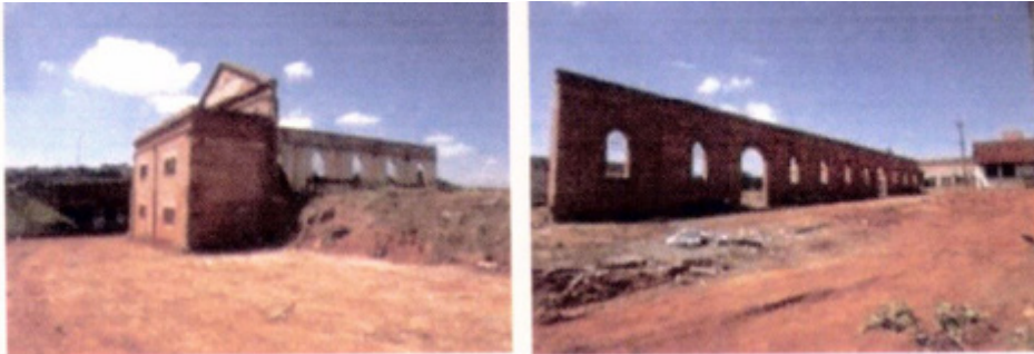
Figures 9 and 10: Views of the remaining masonry.
